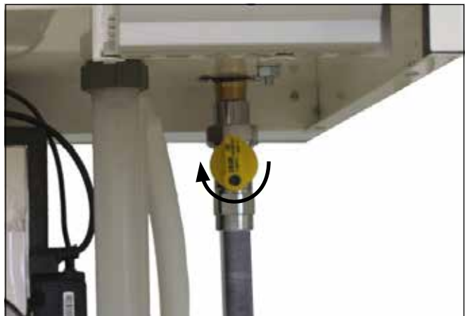
Figure: Gas connection
