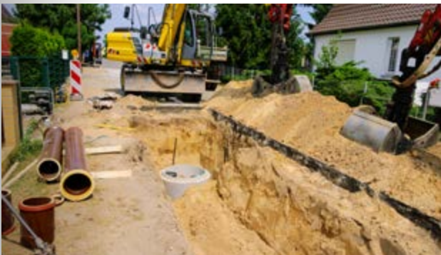
Utilities and services, pipe line and cables
