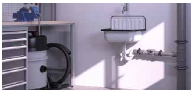
Ø 50 or Ø 75 exposed drainage pipe
